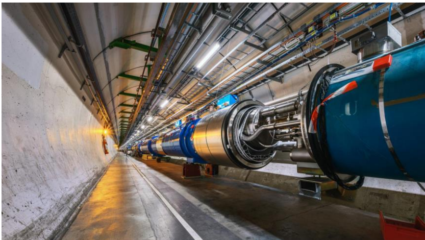
LHC Dipole in Tunnel
