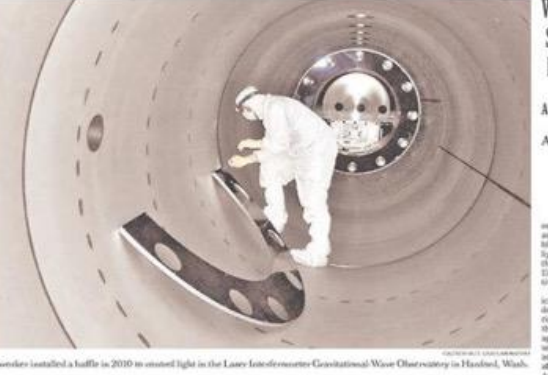
A worker installed a baffle in 2010 to shield light in the Laser Interferometer Gravitational-Wave Observatory in Hanford, Wash.
