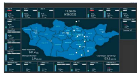
FIGURE III. SCADA DISPLAY OF "TELEVISION" SUBSTATION
