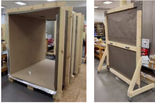
Fig. 6. View of the construction of the EMC test chamber with an external metallic shield installed (the chamber during its construction) and the door of chamber on the right.
