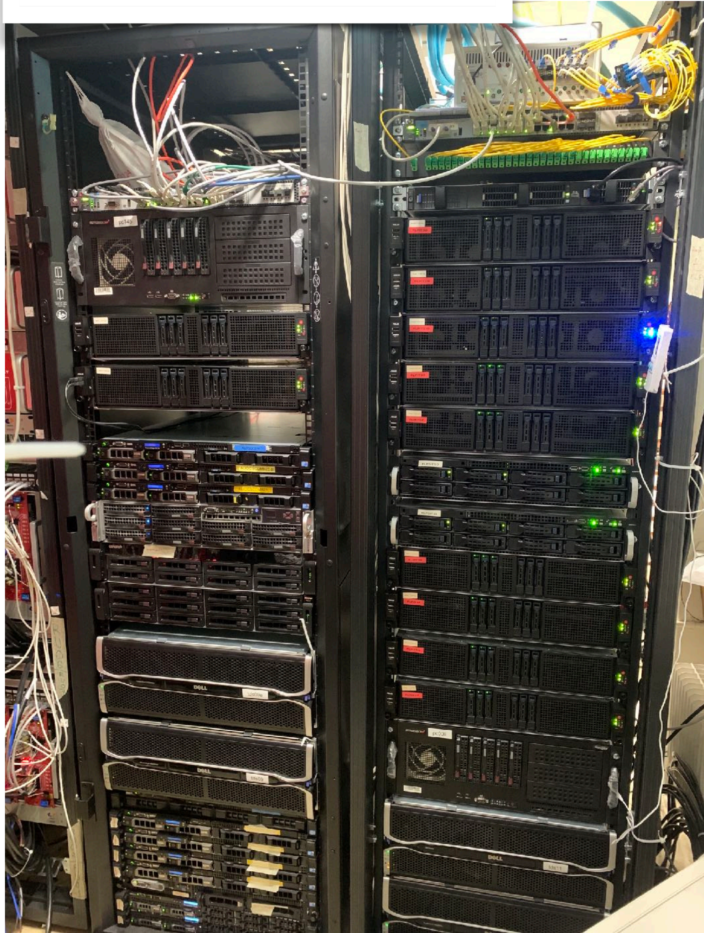
Readout / Control Servers
