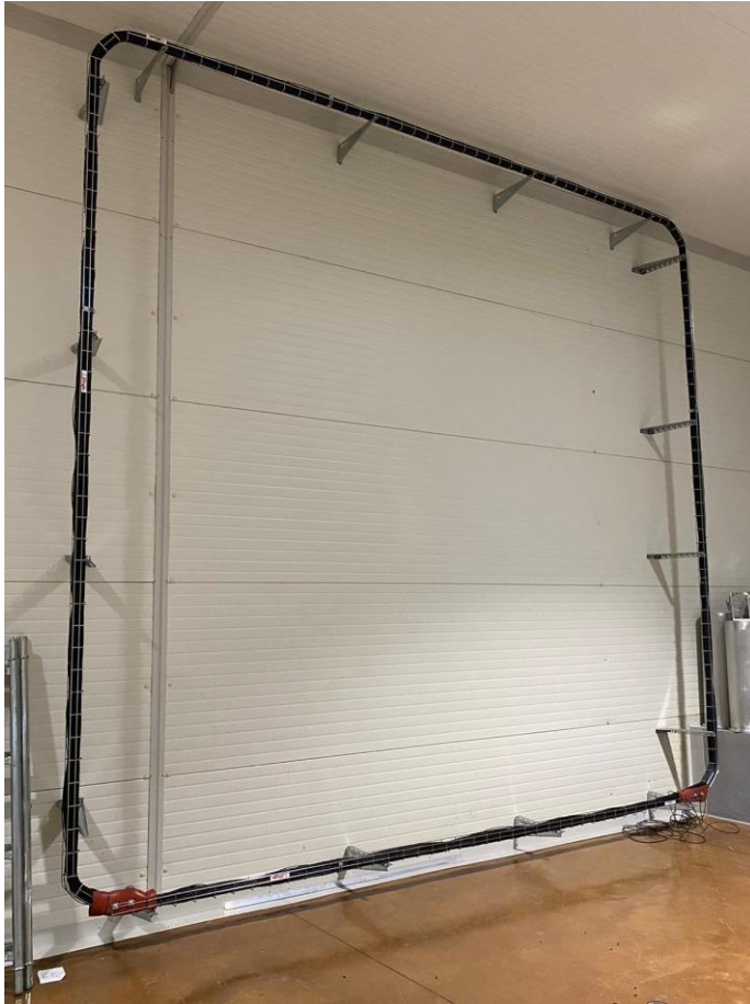
Figure 1. The coil of height 4.2m and width of 4.5m, with 86 loops.
