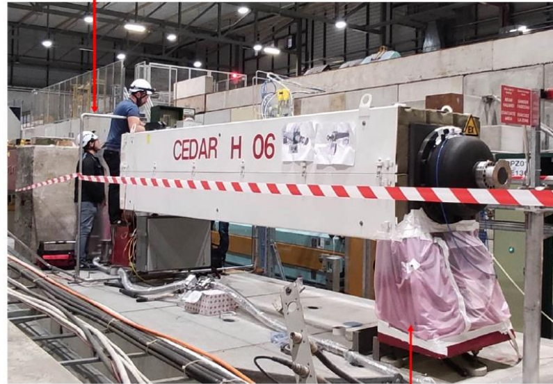
Isolation of motor controls within ATEX zone
