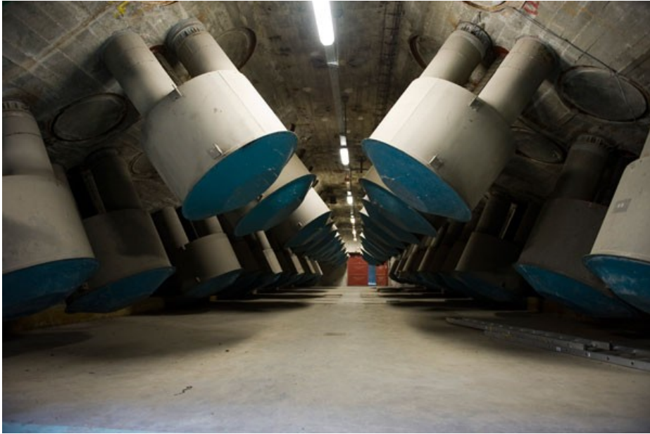
View below the reactor
