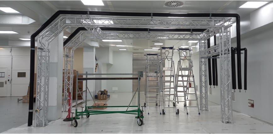
Cooling & Environmental: CO2 for staves, C6F14 for PP2, Dry air to -60°C DP, H&T sensors
