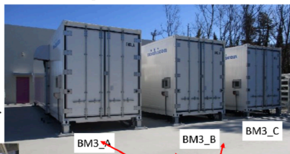
Capacitor Banks for BM3
