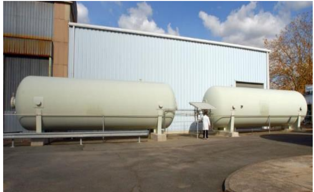
2 x 100 m 3 for a 150 l/h liquefier : - Redundancy for maintenance (PED)
