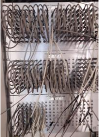
DAQ patch panels
