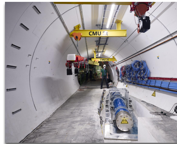
FASER installation in T112 tunnel
