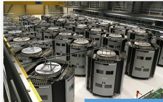
New RF amplifier towers
