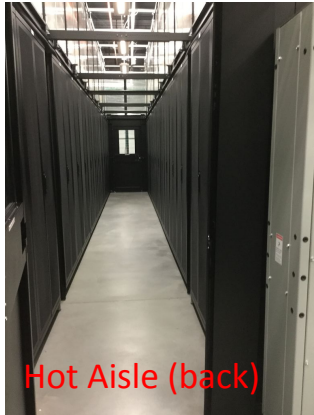
AGLT2 Rack@MSU DataCenter
