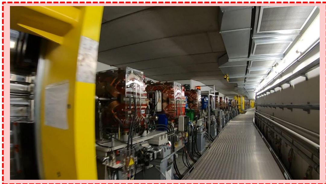
Max von Laue Experimental hall: Double Bend Achromat cell structure and undulators for photon beam production
