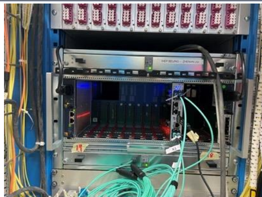
Set up in CMS Underground Service Cavern
