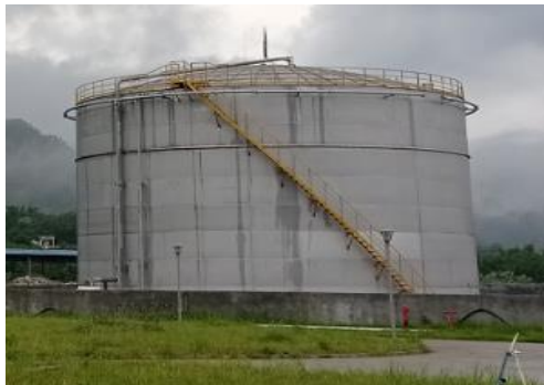
5000 m 3 LAB storage tank
