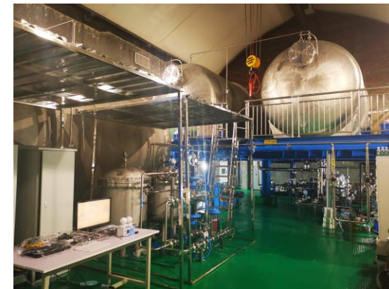
LS filling Control room
