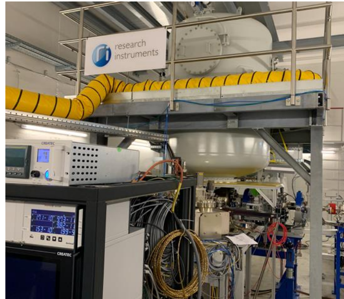
HV power supply suited for high bunch charge (designed for 40 mA, 450 kV)
