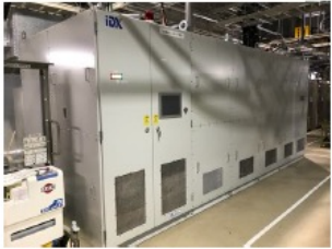
New Horn PS/trans/ strip-lines for 320kA & 1Hz
