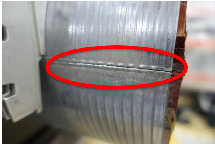
Collaring sheets are collapsing inwards
