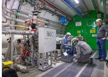
Beam Gas Curtain(BGC) installation in the LHC
