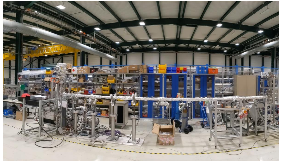
HL-LHC in-situ a-C coating test bench
