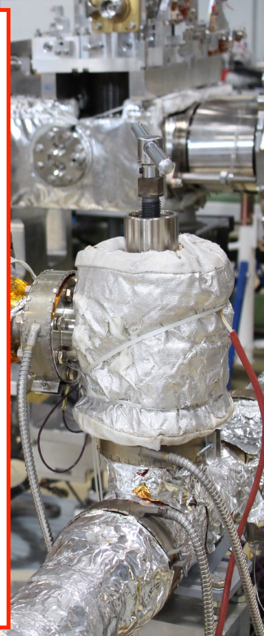
Collimators connected to the UHV test bench: preparation for bake out at 250 °C.
