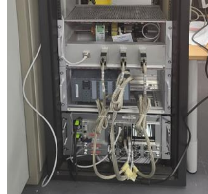
Low Level controls
