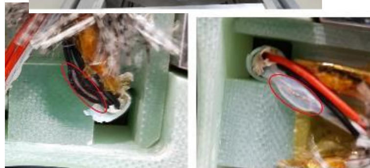
Figure 10 – V-strip exposed conductor
