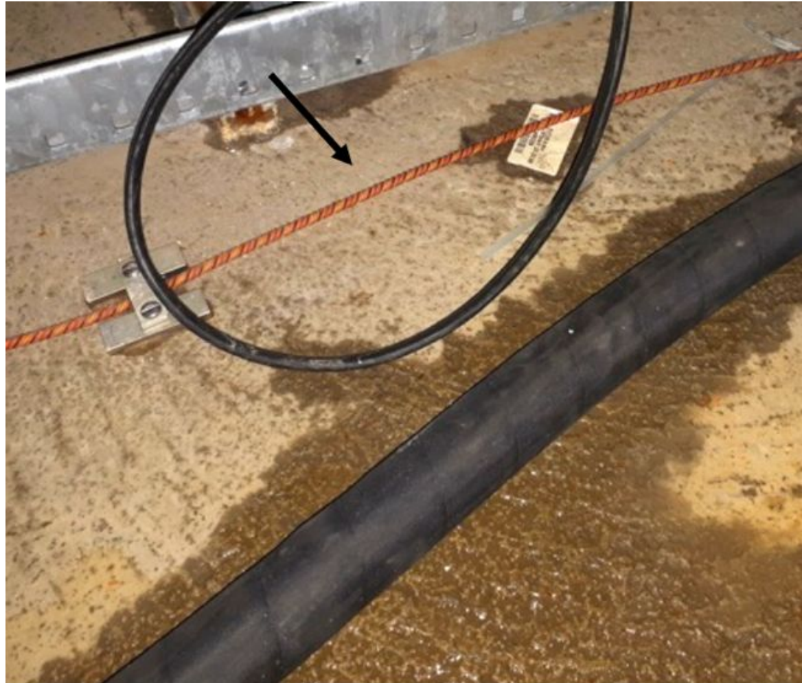
Sensing wire near leak
