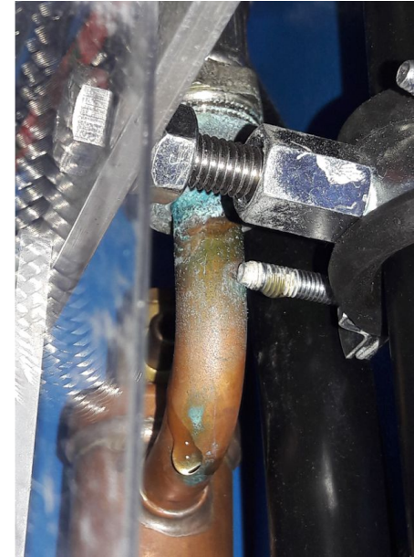
Small leak inside rack
