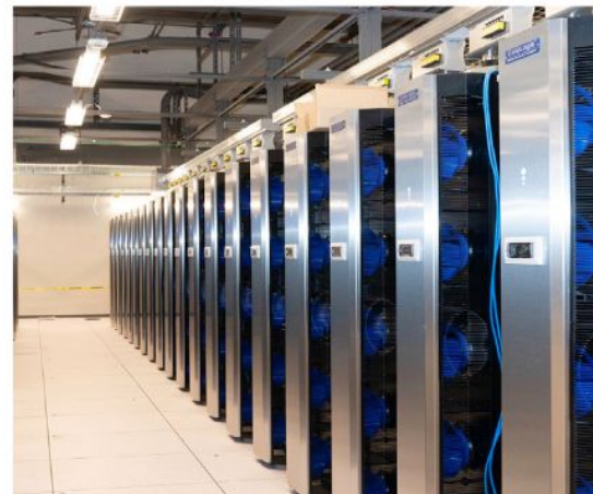
Tier 1 center in new building at BNL
