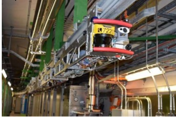
Train Inspection Monorail (TIM) for inspection & RP measurements in LHC
