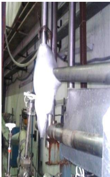
Return line leaks
