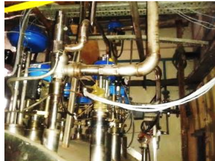
Safety valve with NRV in system
