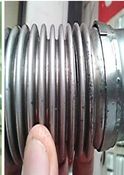
Crack in Bellows
