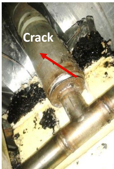
Dish end crack
