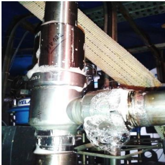
Leakage in safety v/v outlet
