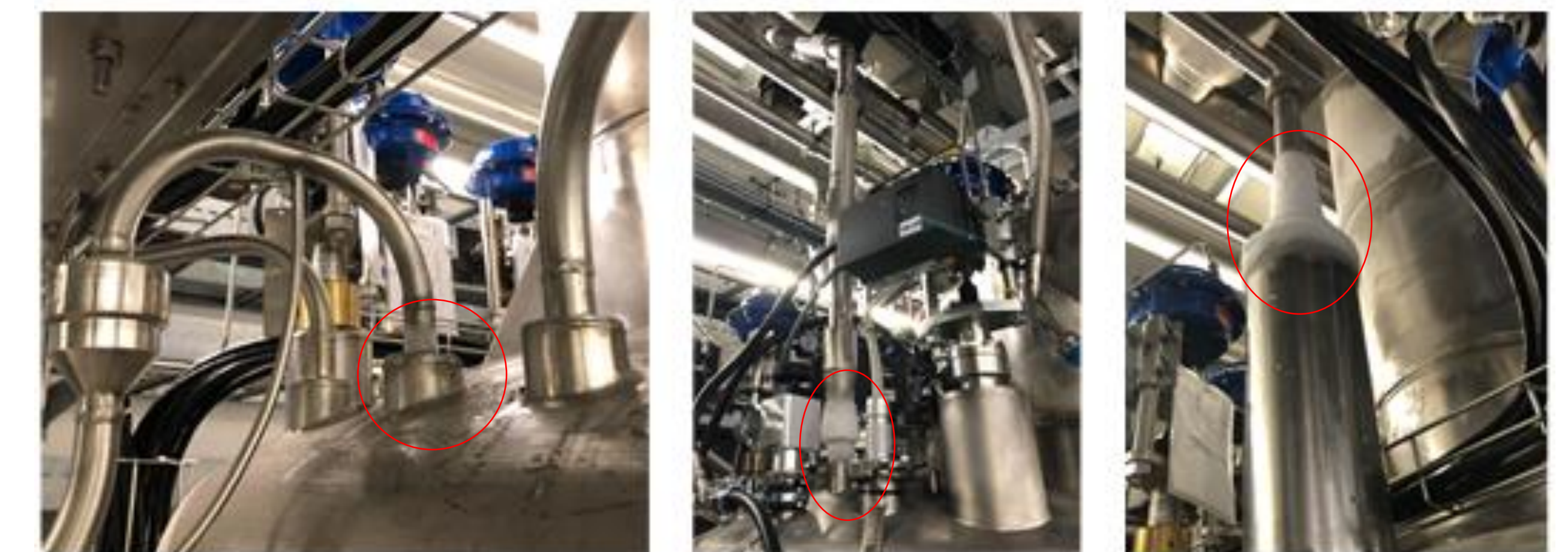
Cold spots due to valve seat leak from cold side to warm side
