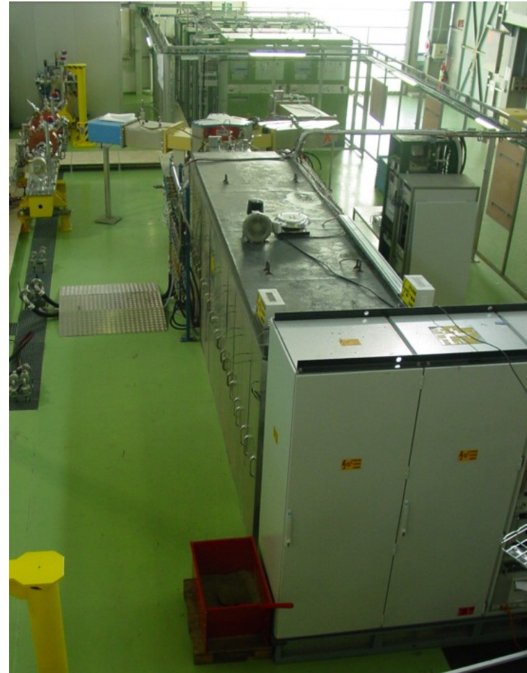
LEP-type klystron and prototype modulator under test
