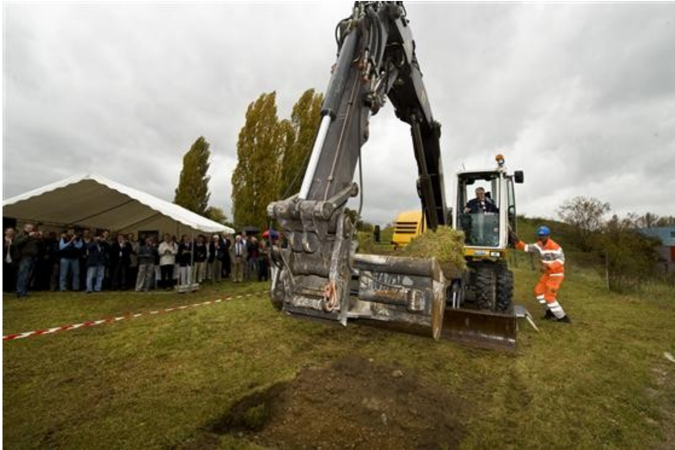
Groundbreaking (and start of civil engineering works) 16.10.2008 1 year 4 months after approval of the project
