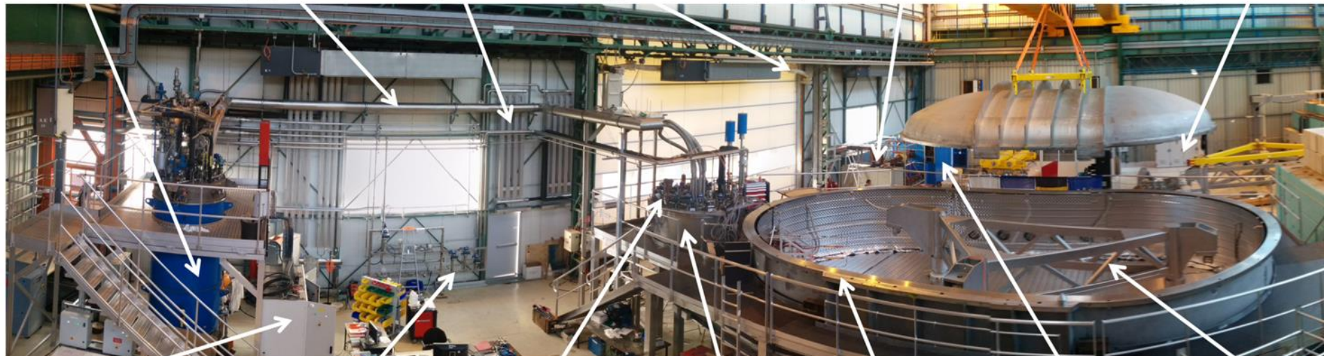
Process and control cabinets Warm valves HTS current lead Valve box Cryostat Power supply Test frame
