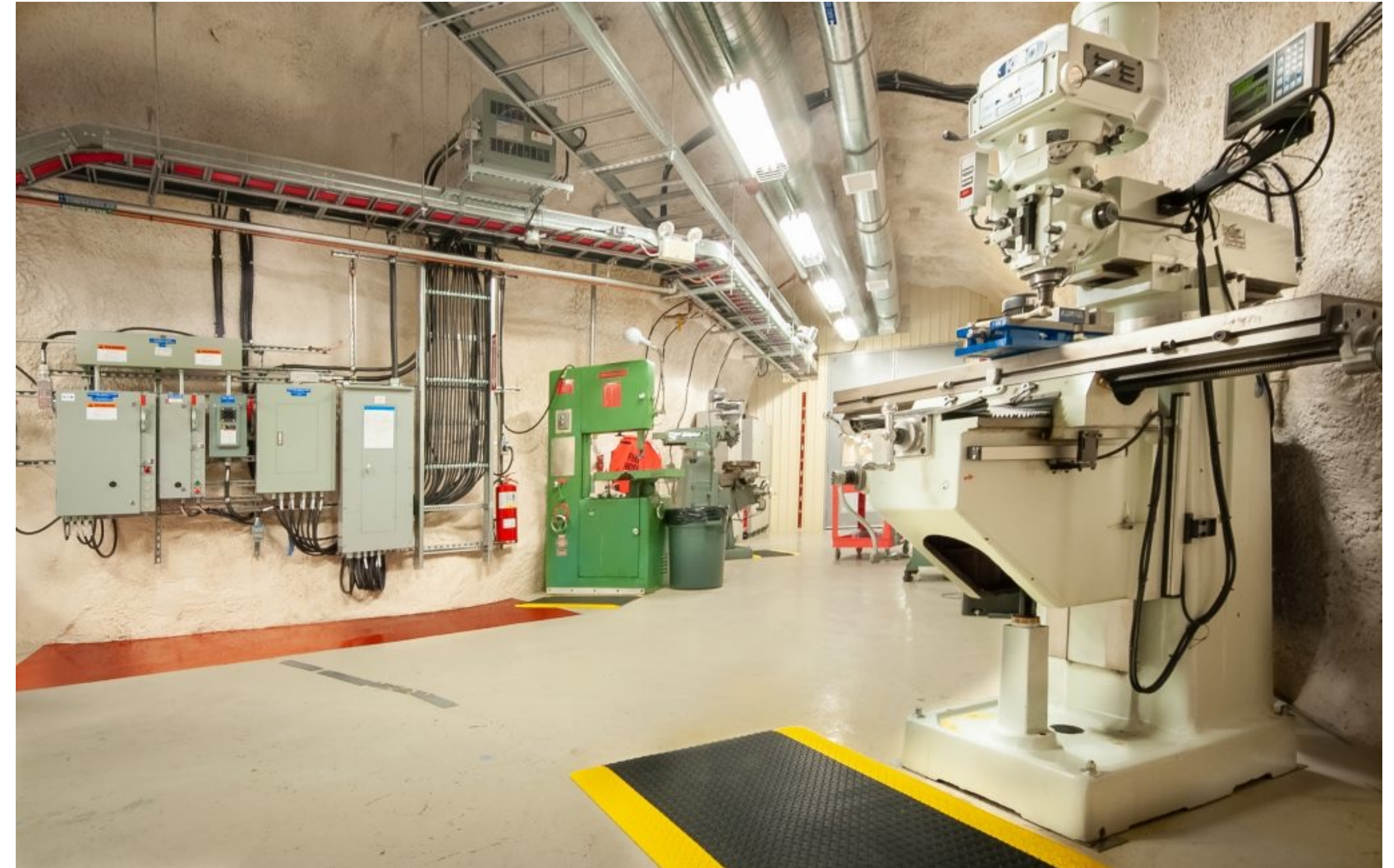
Underground Cleanroom Machine Shop in SNOLAB
