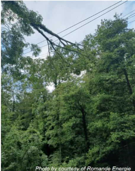
Photo by courtesy of Romande Energie
