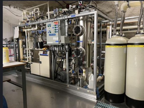
Underground UPW Assay System
