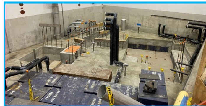
Target hall shielding
