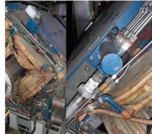
Consolidation of final focusing quadrupoles (QDE209, QFO210, QDE321, QFO322)
