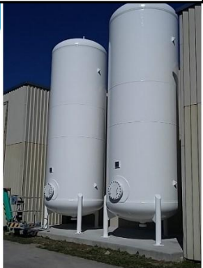
Helium gas storage
