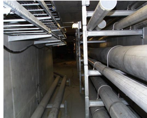
Industrial stainless steel piping
