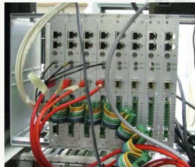
Back side of SRS FEC interface
