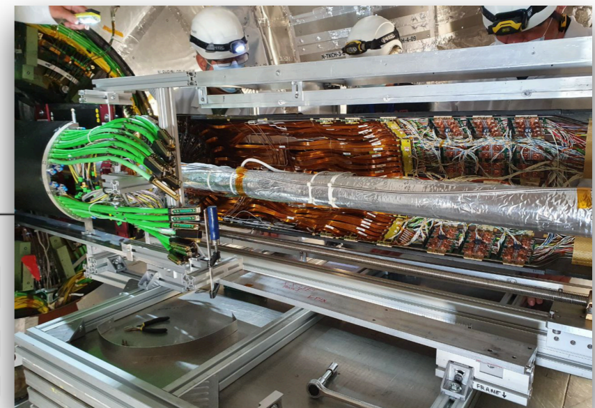
FPIX insertion with service cylinders (4 pieces, 2 per end)
