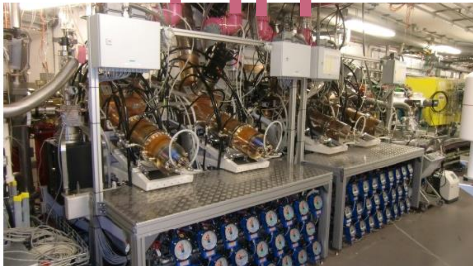
500MHz Cavities at BESSYII
