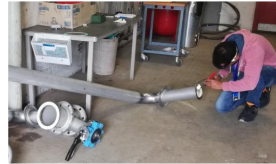
Direct visual on piping weld, cooling water circuit in CERN BA4
