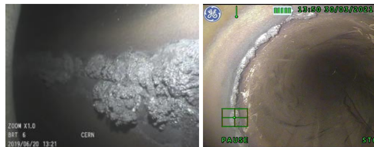
Weld root porosities observed in narrow access (LHC MB diode box) and large pipe (He recovery line) situations require different probe size and tip optics
