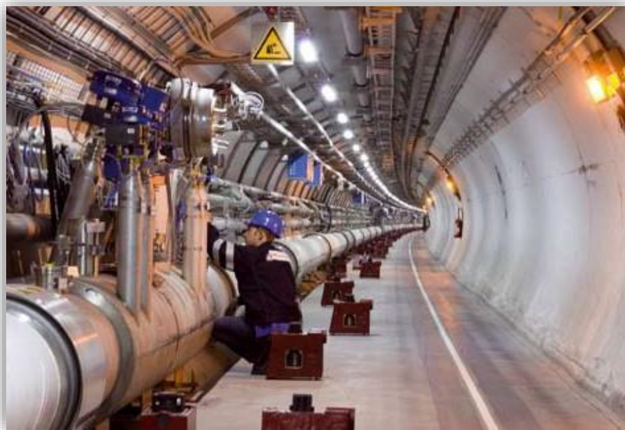
LHC He transfer line (before magnet installation)
