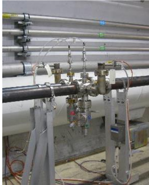
A measurement & pumping port
