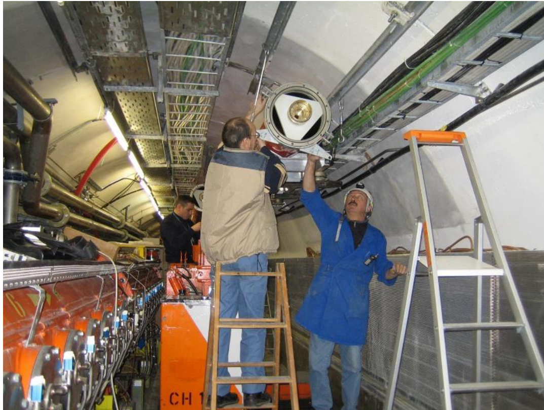
345 mm Coaxial Line Installed suspended from the ceiling
