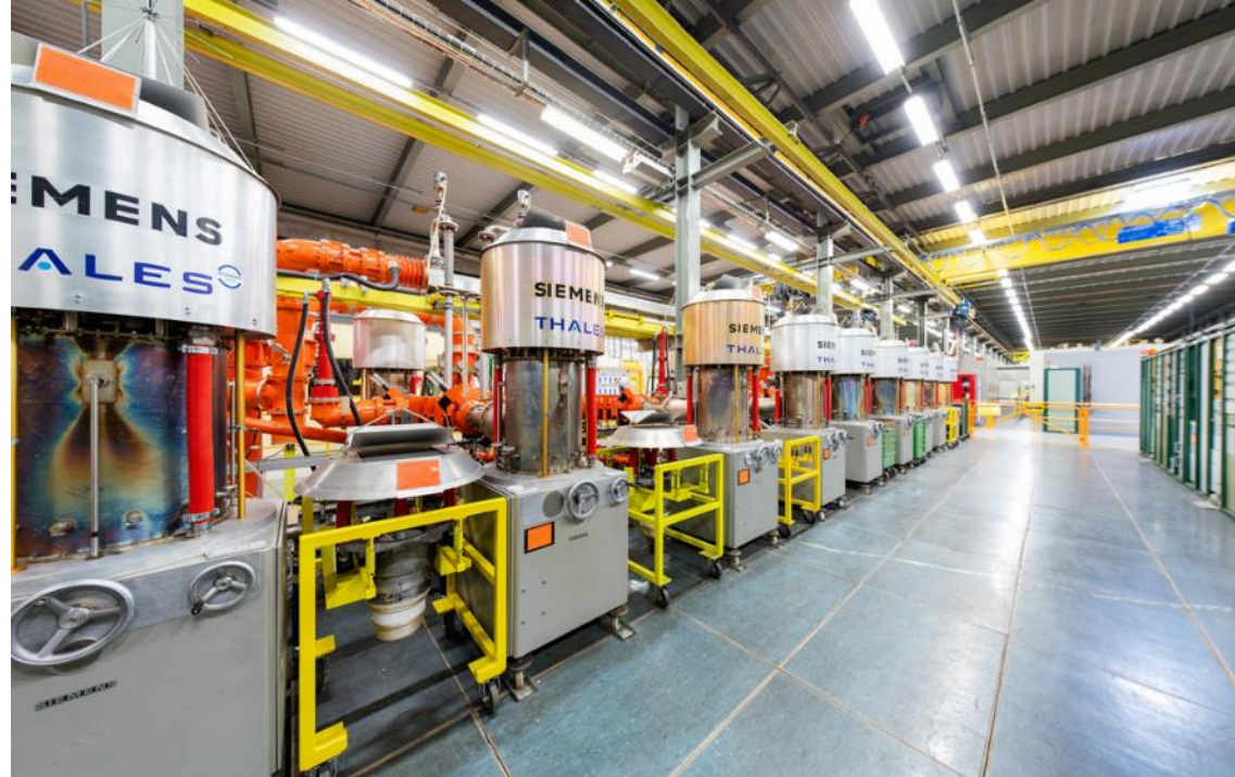
CERN SPS 'Siemens' Power plant 2 x 600kW continuous wave @ 200MHz Based on RS2004 water cooled tetrodes In operation since 1976 (almost 50 years ago)
