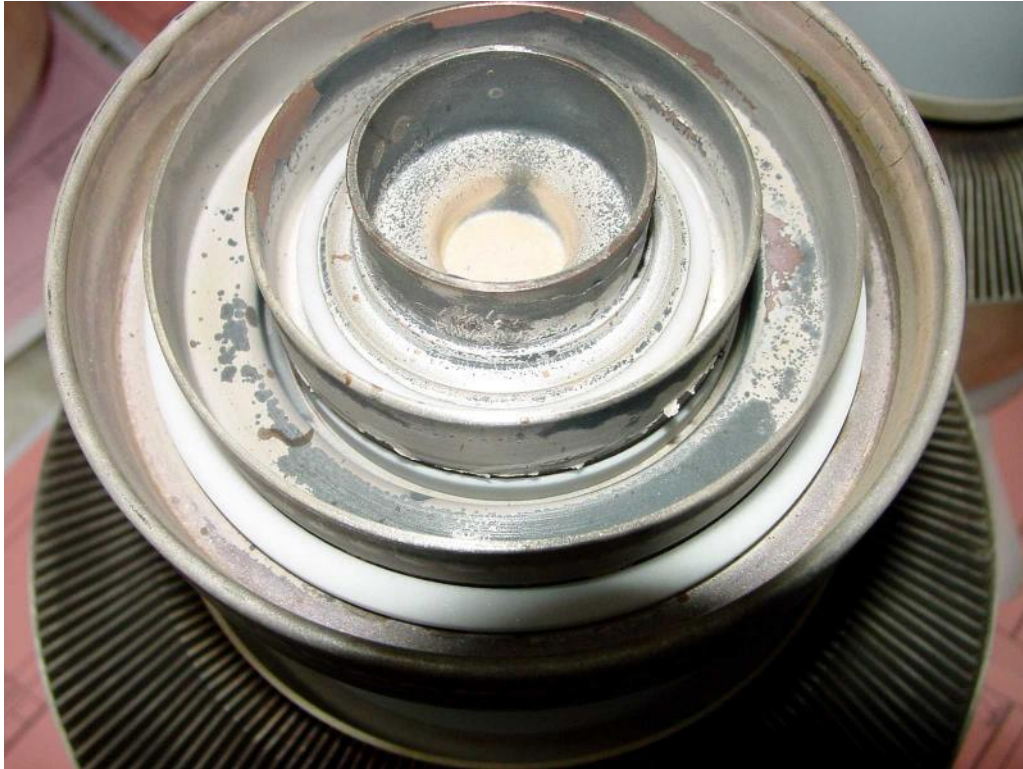
Overheating due to lack of air cooling
