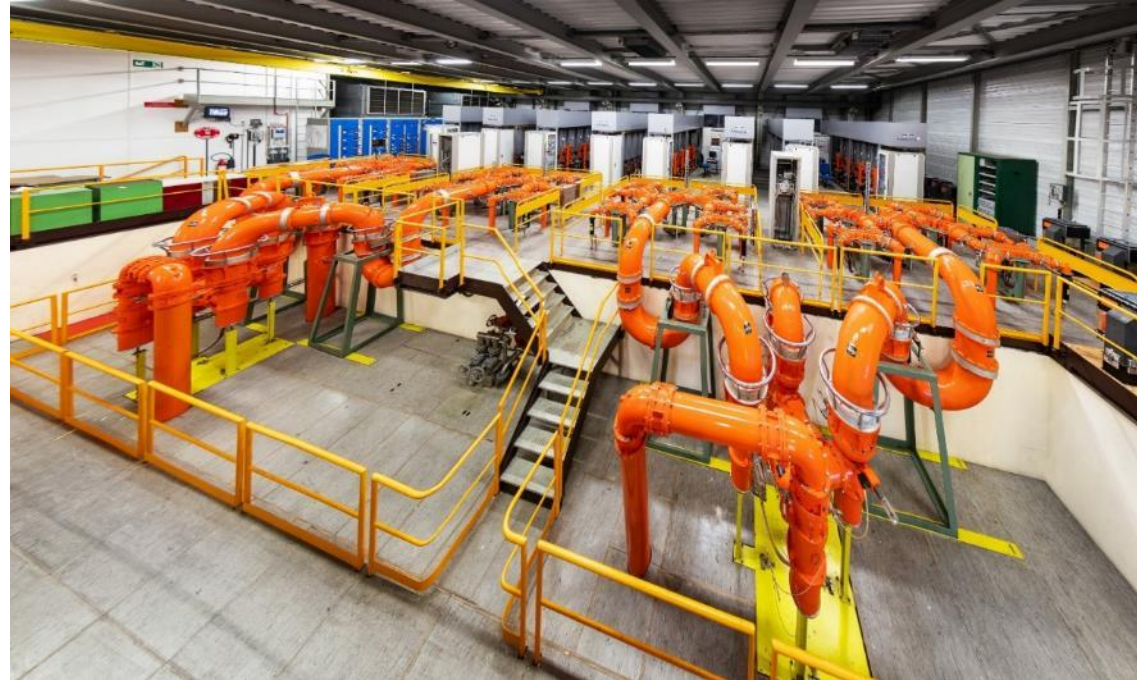
CERN SPS 'Philips' Power plant 2 x 600kW continuous wave @ 200MHz Large 3dB combiners In operation since 1981 (more than 45 years ago)
