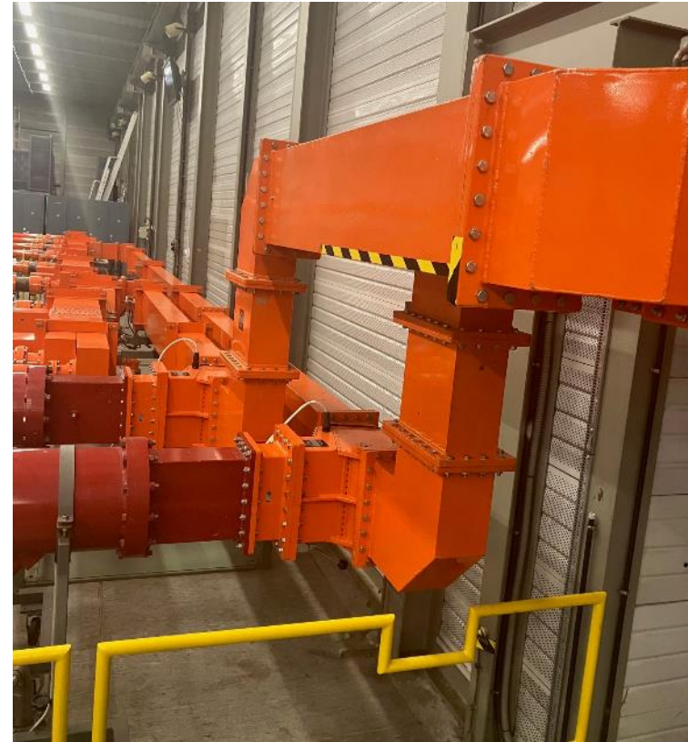
CERN SPS 'Electrosys' Power plant WR1150 waveguides operating @ 800MHz 3dB combiner, rotative switch, elbows and straight lines In operation since 1989
