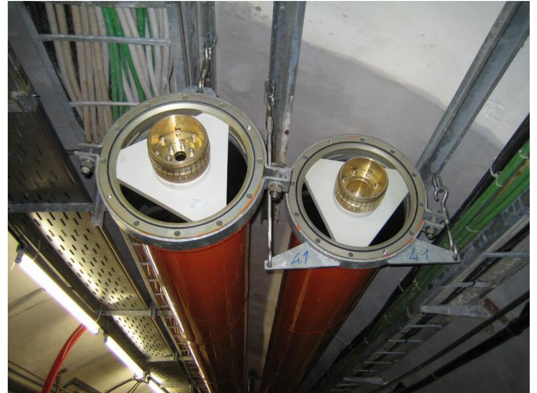
The supporting system is made to allow for movements due to thermal expansion
