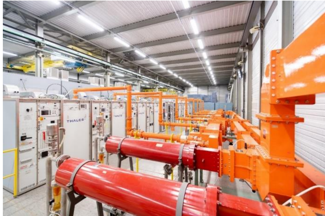
CERN SPS 'Electrosys' Power plant 2 x 160kW continuous wave @ 800MHz Based on IOTs In operation since 2013 (more than 10 years ago)
