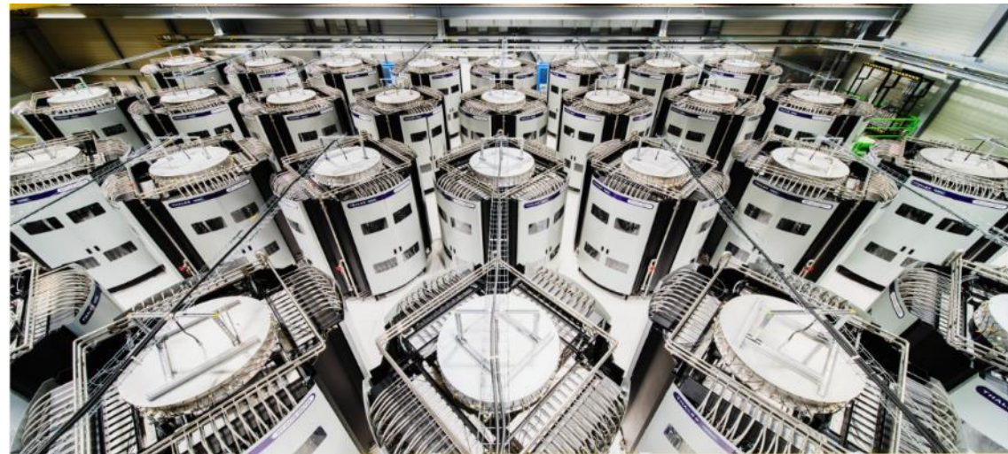
CERN SPS 'Thales' Power plant 2 x 800kW continuous wave @ 200MHz Based on Transistors In operation since 2021 (a few years ago)
