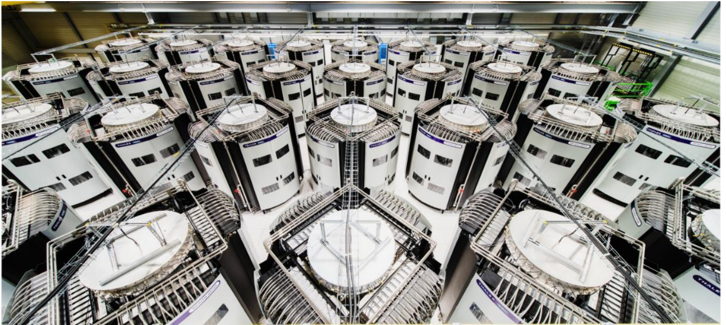
CERN 2 x 16 x 160 kWp @ 200 MHz tower solid state amplifiers (2021)
