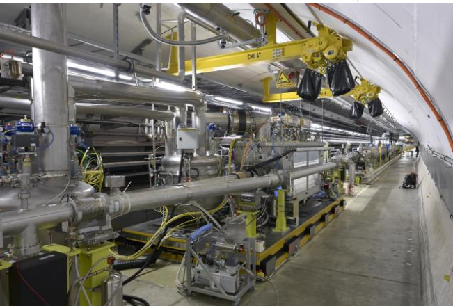
Support with mobile Y-chamber for the crab cavity test stand in SPS
