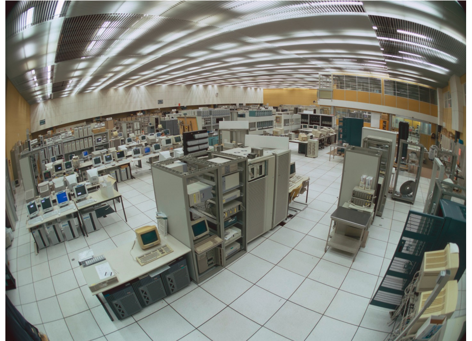
CERN Computer Centre around 2001
