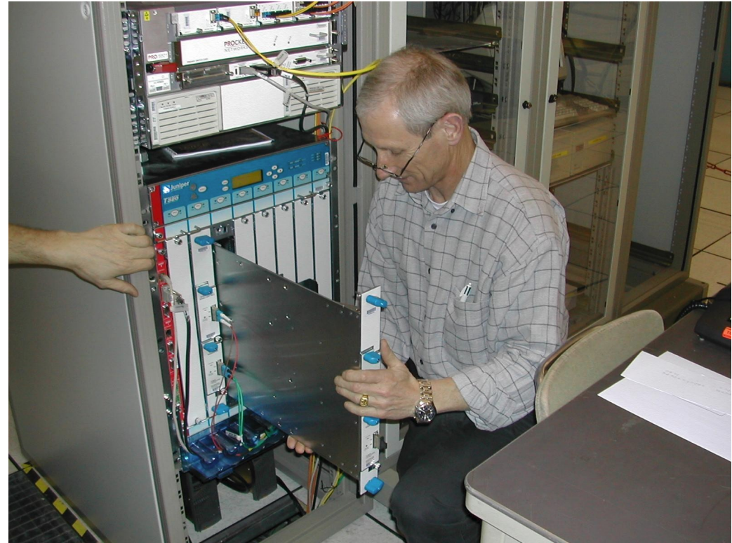
Martin Fluckiger (IT-CS-EN) install a linecard on a brand-new Juniper MX router.
